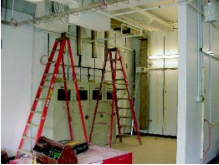
Figure 2: Hutch G-3 under construction. Exhaust stacks are being connected between the two ladders to the 4 gas cabinets that house containers that will feed reactive gasses into the real-time growth chamber (not yet installed). The front lead and steel hutch doors are not yet in place.
